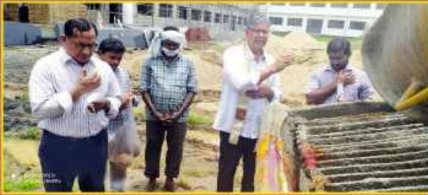
Fr. Sandanasamy blessed slab for water tank in the New Primary Block
